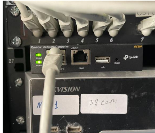
The OC200 in network cabinet.
